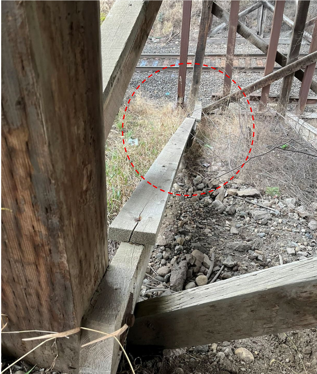
Figure 2-1: Bent 4 columns had no signs of decay however there is a small soil failure around column 5 that is causing the column to displace a small amount. This displacement is also evident in the bottom longitudinal bracing which has a bend in the brace between bents 3 and 4.
