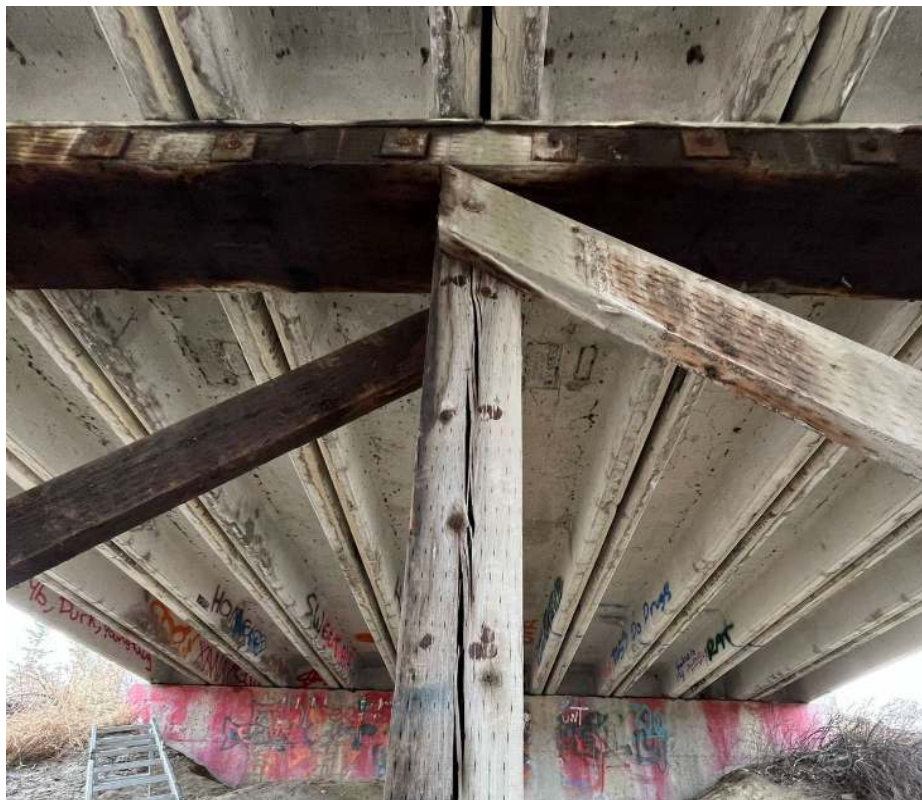
Figure 2-3: Bent-1 Cap shows water stains and degradation.
