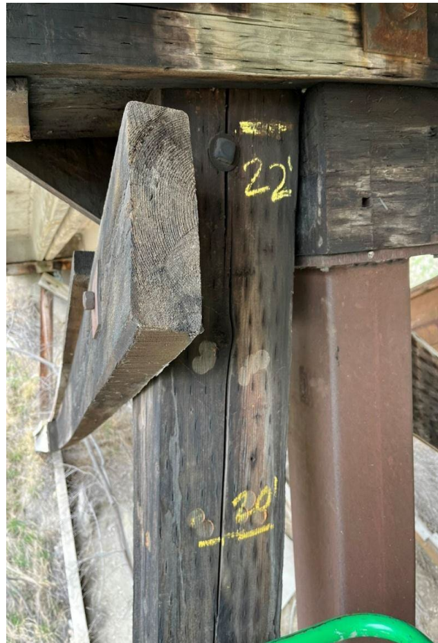
Figure 2-14: Bent 3-Column 1 shows a split at the bolt location extending along its length.
