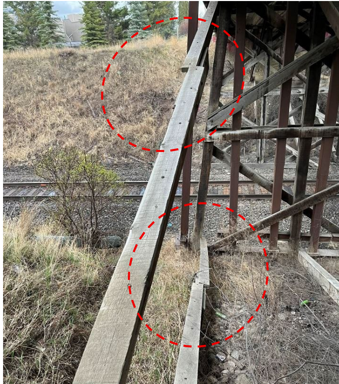
Figure 2-2: Longitudinal bracing between Bents 3 and 4 east side (adjacent to Column 5), showing deformation/loose connection in the brace members.
