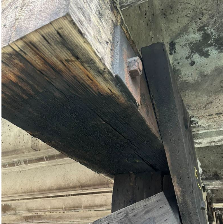
Figure 2-17: Bent 2 bottom of cap shows high moisture content.
