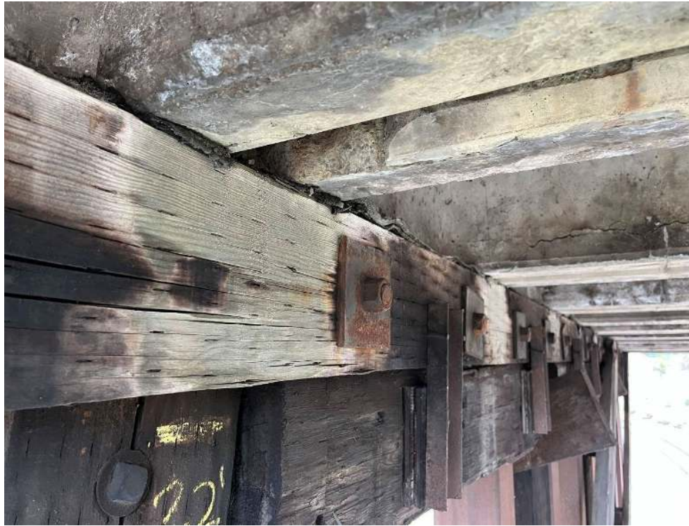
Figure 2-4: Bent 3 cap shows signs of water leaking from the superstructure.
