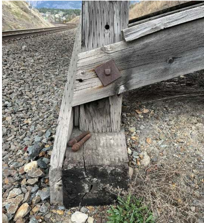
Figure 2-6: Bent-2 sill shows degradation.
