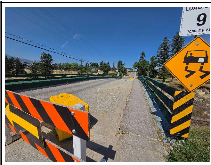
Photo 4: Hazard of note includes blocking traffic when working on renovation of bridge
