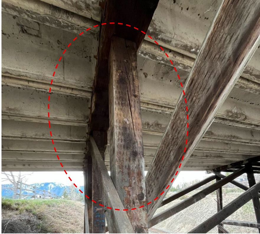
Figure 2-9: Bent-1 Column-4 exhibits wide checks. Enhanced by vertical drift pinning and subsequent decay in the top of the column.
