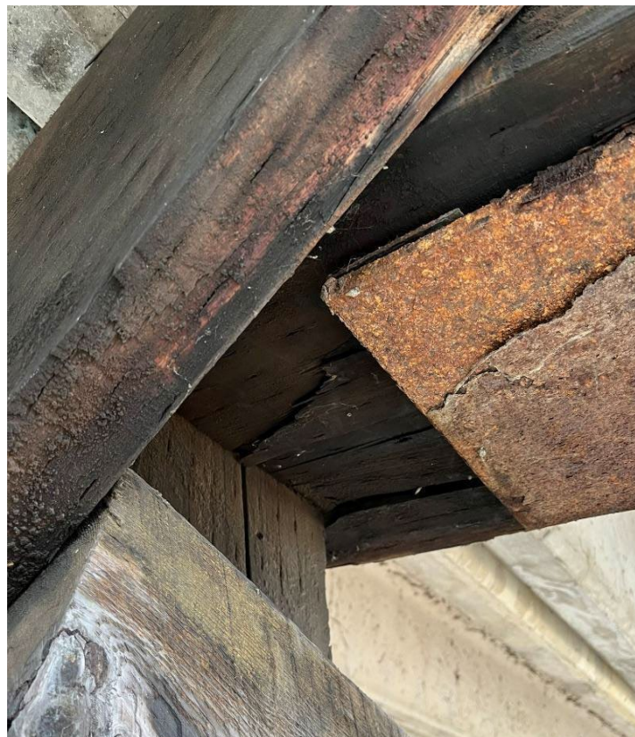
Figure 2-7: Bent 3 cap, steel plate is severely corroded, creating a gap between the timber and steel and compromising bearing.
