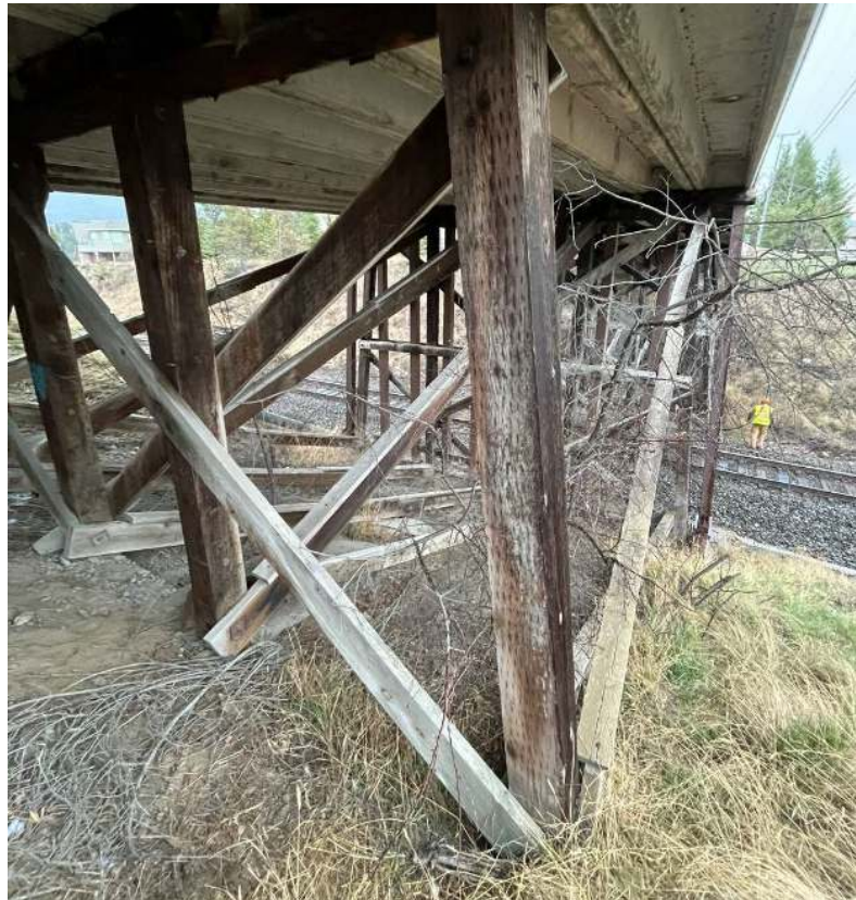
Figure 2-20: Build-up debris between Bent 3 and Bent 4.
