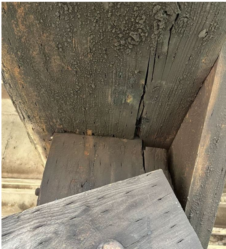
Figure 2-18: Bent 2 Column 5 split at top of column and cap is decayed.
