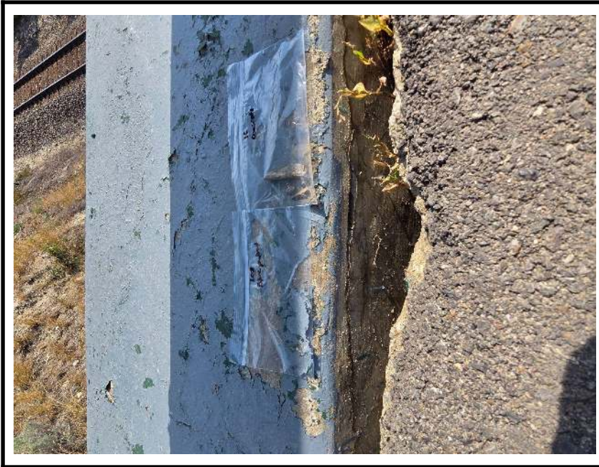
Photo 3: Light blue paint sampled in the Project Area (Central Bridge) contains 147 µg/g of lead
