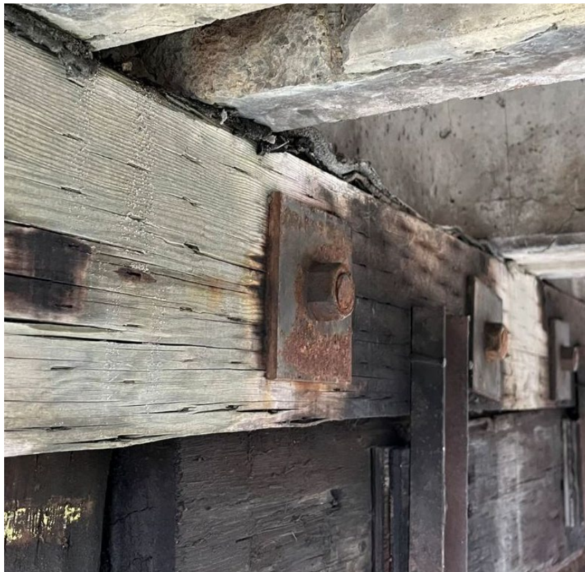
Figure 2-5: Fasteners and plates show signs of corrosion.
